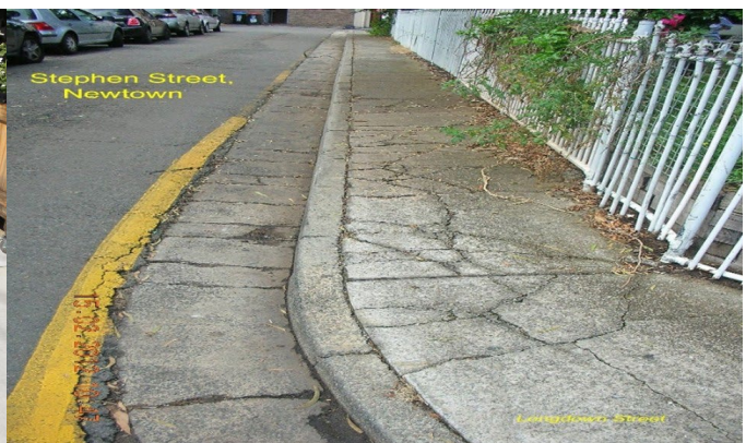
Condition 5 – Very poor
