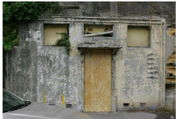
Condition 5 (very poor)
