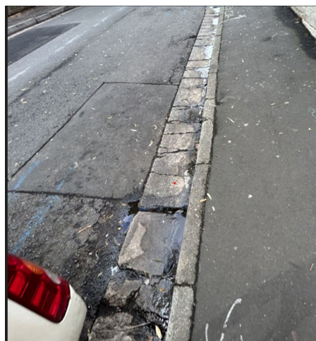
Condition 5 – Very poor
